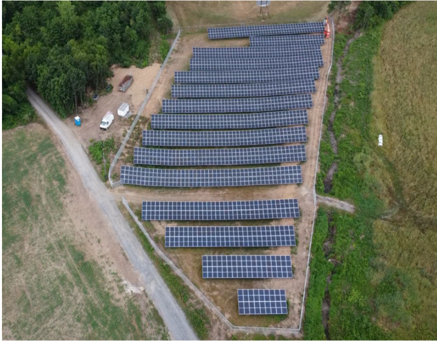
West Snyder Elementary School 460KW
