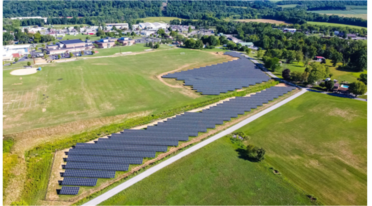
Behind the High School 2.1 MW Bifacial panels
